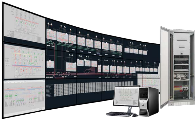
3 rd level. Operator control
