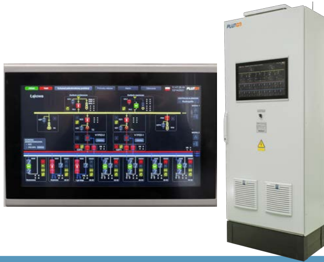
2 nd level. Substation control
